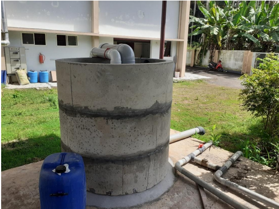
Fig. 4 Tank for collecting the rainwater from roof
