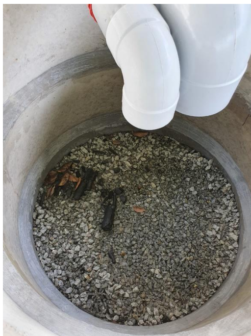
Fig. 5 Filtering techniques used in the tank for collecting the rainwater from roof
