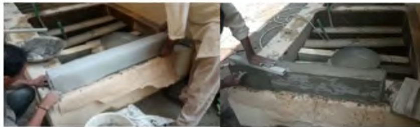
Fig8. Application of AR glass mesh Fig 9. Application of mortar over the layer
