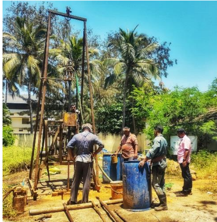
Photo#7: Soil investigation work at Library and Reading room for Kochuveli St. Joseph Library
